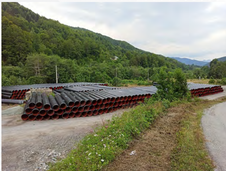
Photo: Vuk Vujisić, Water pipes on stock at Bara Kraljska construction site
